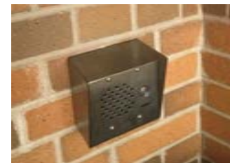
Intercom Box at Main Entrance
