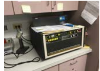
Intercom System Head-End
