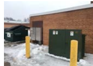
C/T Cabinet & Utility Transformer
