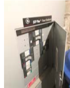
Main Electric Service
