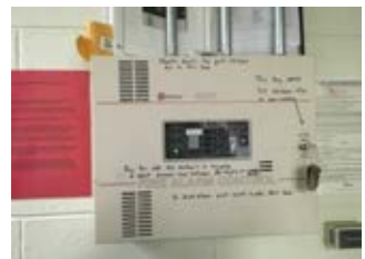
Fire Alarm Control Panel
